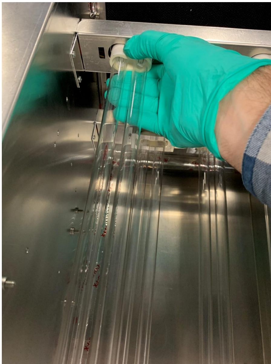
Figure 13: Remove all Four Old Bulbs by Carefully Pulling on the Ceramic Base
