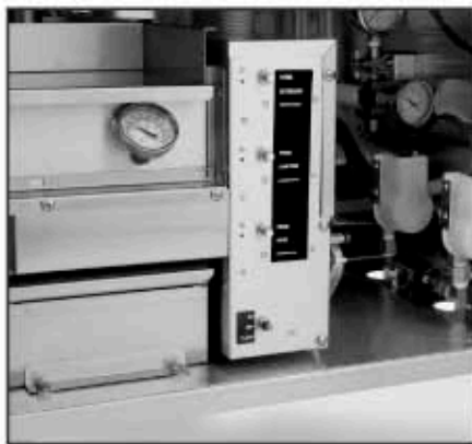
Interior controls provide easy access for changing chemical settings and service.
